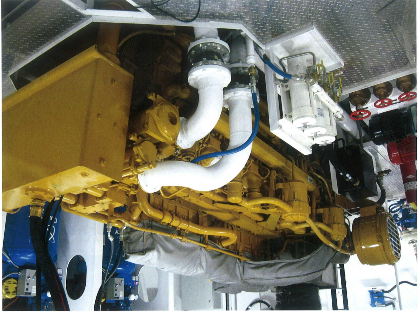
Two Caterpillar 3516 Tier 3 propulsion engines each produce 2,575 HP at 1,600 rpm, and maintenance is simplified by several innovative features from the yard including main engine filters located at floor level beside the engine in a tray to contain drips and bilge pump valves clustered under the ladder in a cutaway in the floor. Photo by Peter Marsh.
